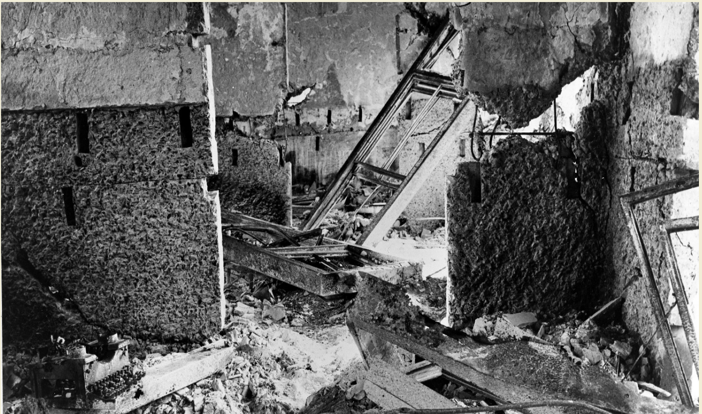
NARA Archives Catalogue, Room Content Destroyed By Fire, NAID: 134403973, Local ID: 243-R-2-32
